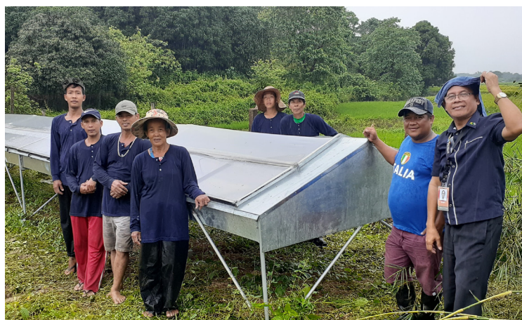
MPC members and Dr. Capariño are at the on-going construction site of their office and processing area.
